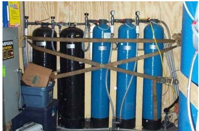
Camp Edwards Ion Exchange Test Container
